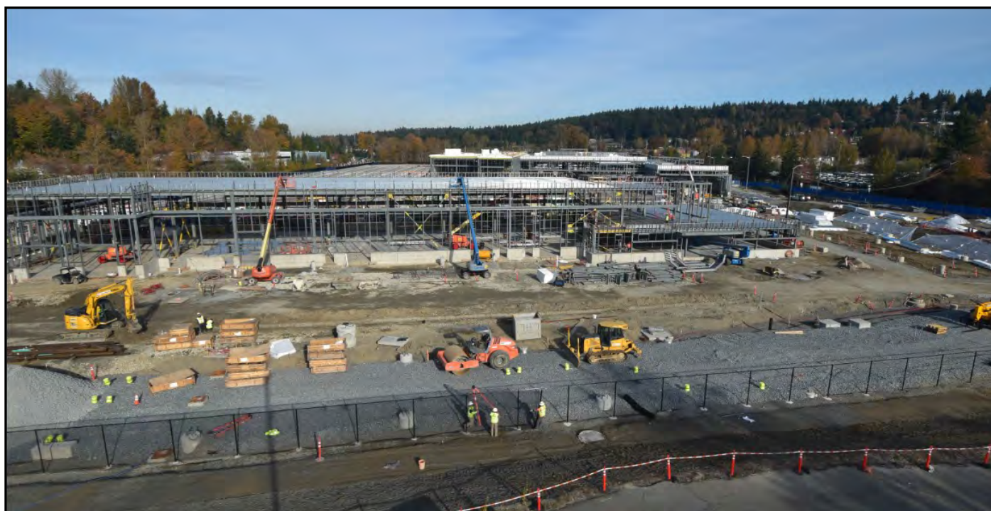
OMF East looking north taking shape with yard scope and steel structure framing on October 31, 2019
