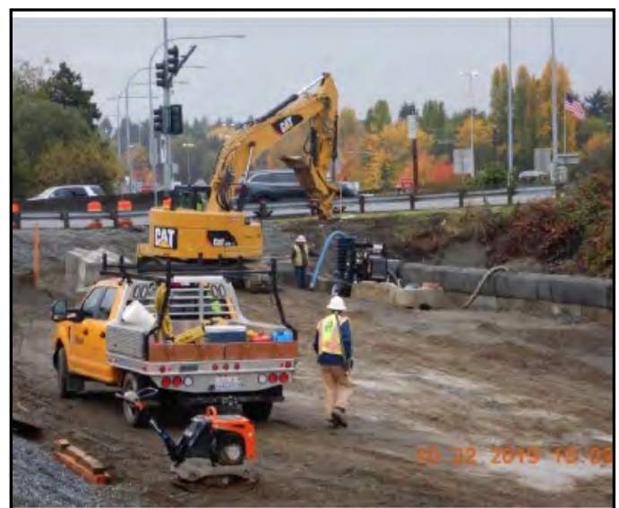
WZ-1 Northgate Pond pumping to Basin A
