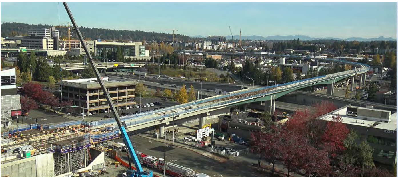
E335 Downtown Bellevue to Spring District: Bridge spanning over Highway I-405 along NE 6th Street on October 31, 2019
