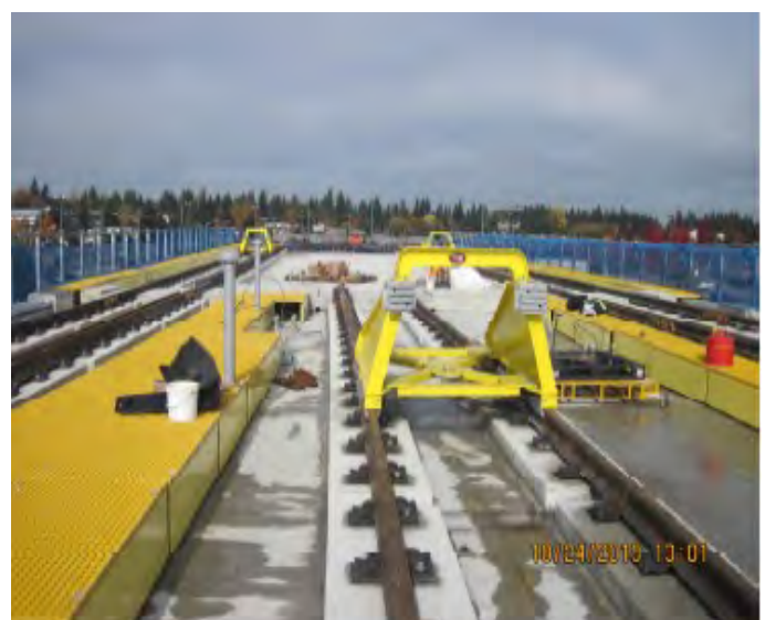
Crew install bumping post at north end of the pocket track in Work Area 7.2
